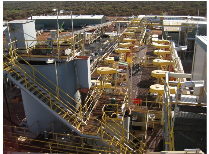
Processing Plant at the Magellan Metals Mine near Wiluna
